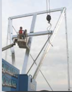
Ironworkers with Majestic Steel Erectors, Inc., Shorewood, IL, make final connections and adjustments to the 40-foot steel cross-support frame before it is lifted into place atop the 128-foot tower.
